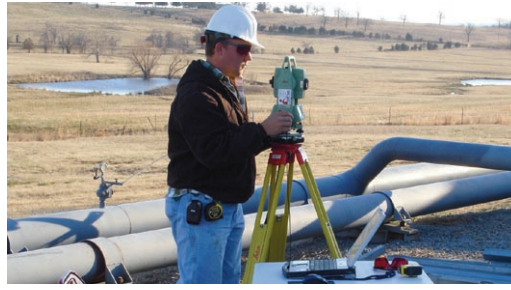
Figure 1. It took two engineers only six months to create intelligent as-builts of 70 compressor stations.
