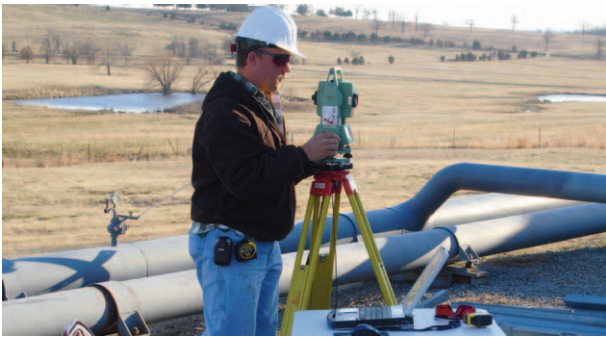
Figure 1. An engineer using a Leica Total station linked to CADWorx fieldPipe to produce on site accurate as built deliverables.
